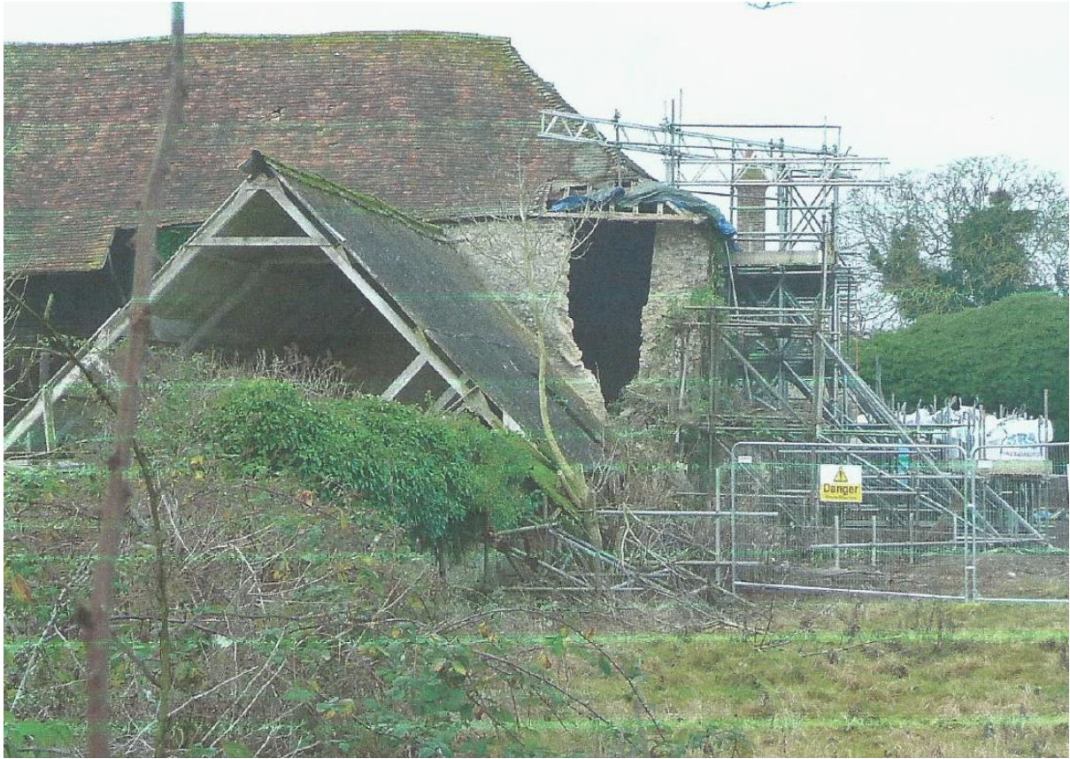
Figure 21: Charing Archbishop's Palace Great Hall, December 2016. The North-East corner has collapsed and the north wall leans out (Charing History Society).
